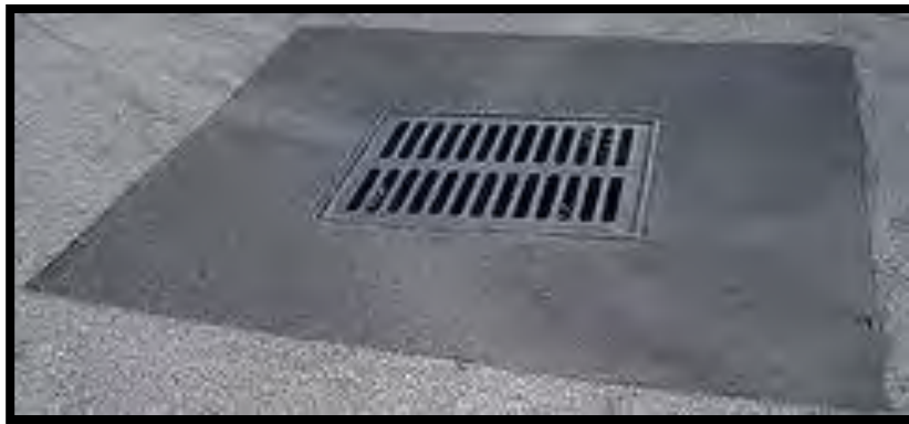
Figure 62. Overhead grate-type road surface covering.
