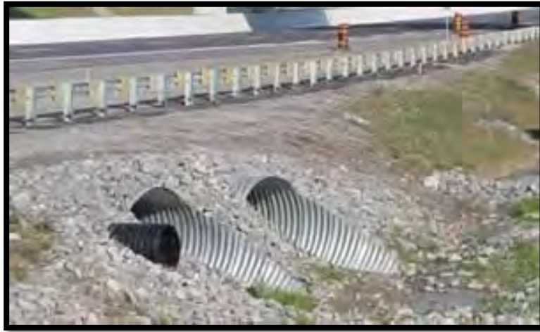
Figure 61. Oversized CSP culvert (Photo Credit: Great Wall Co).
