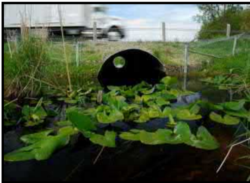
Figure 63. Oversized CSP culvert, partially submerged.
