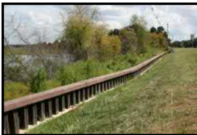
Figure 65. Directional wildlife fence, steel piling (Photo Credit: Aresco MJ).
