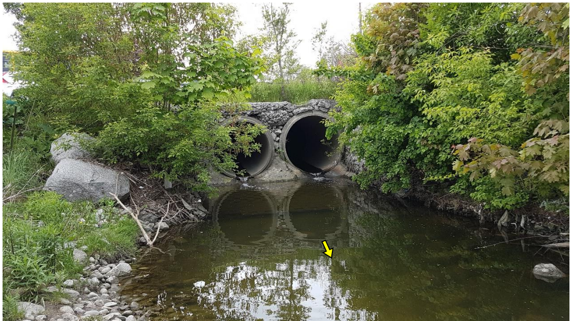
Three perched concrete culverts discharged to the creek downstream of Rutherford Road. The adjoining culverts likely conveyed subsurface storm water drainage from adjacent lots / roadways.
