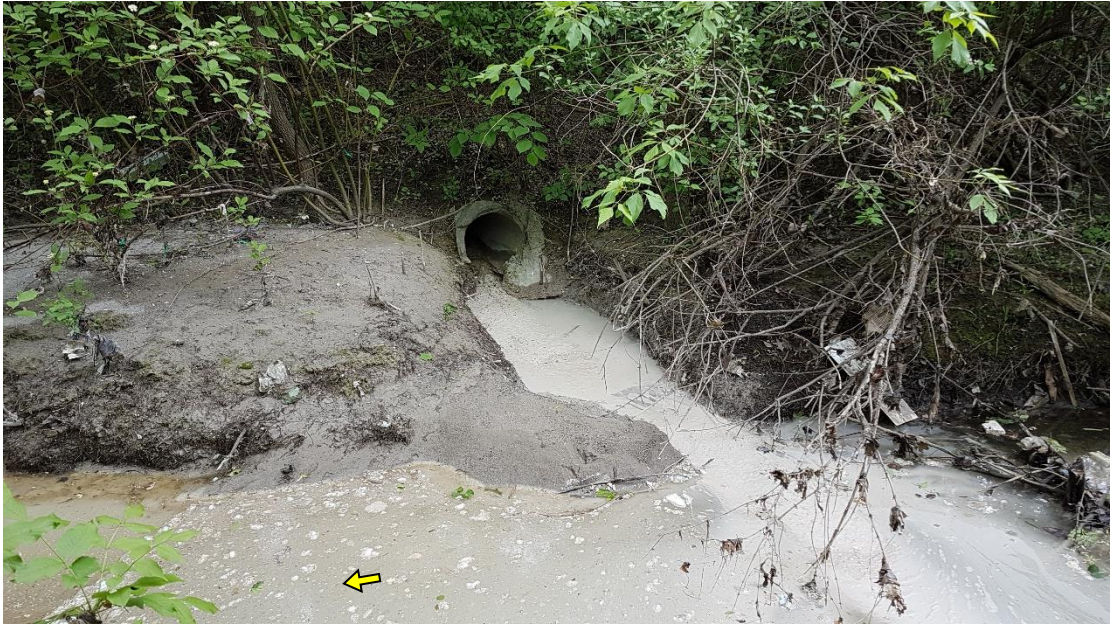
An outlet along the south bank near Rutherford Road discharged a slurry of unknown substance into the creek.
