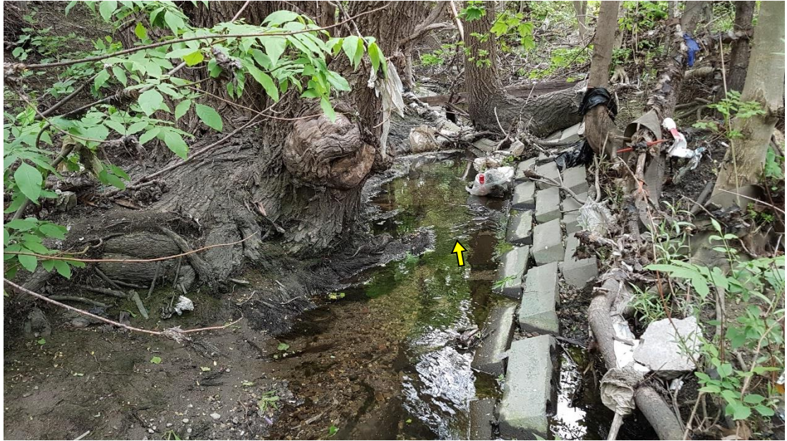
Mature trees had grown over the brickwork and provided indication of the dated nature of the protective treatment.
