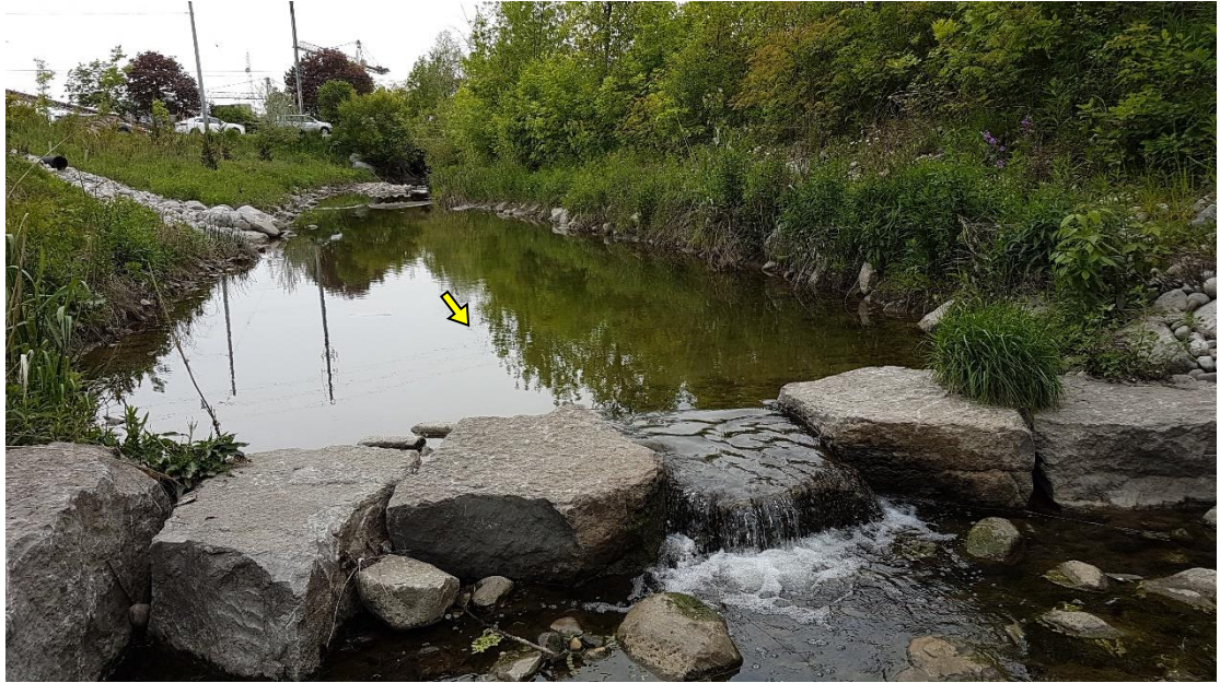
A particularly raised armoursone weir located 65 m from Rutherford Road partially impounded flows and restricted fish passage.
