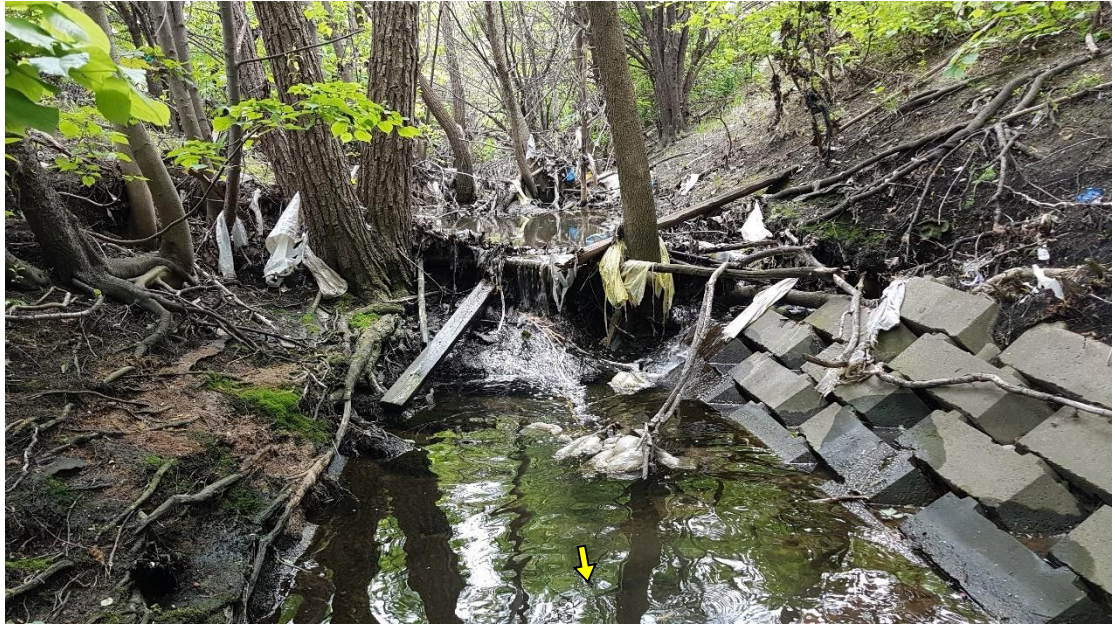
Multiple debris jams were observed throughout the subject reaches, leading to significant aggradation and burial of the brick treatment upstream.
