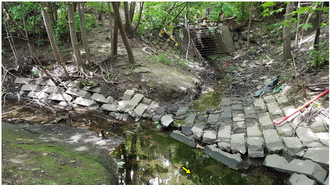
There was a sharp bend in the channel 200 m downstream of Hansen Road, where an adjoining outfall contributed minor flows.
