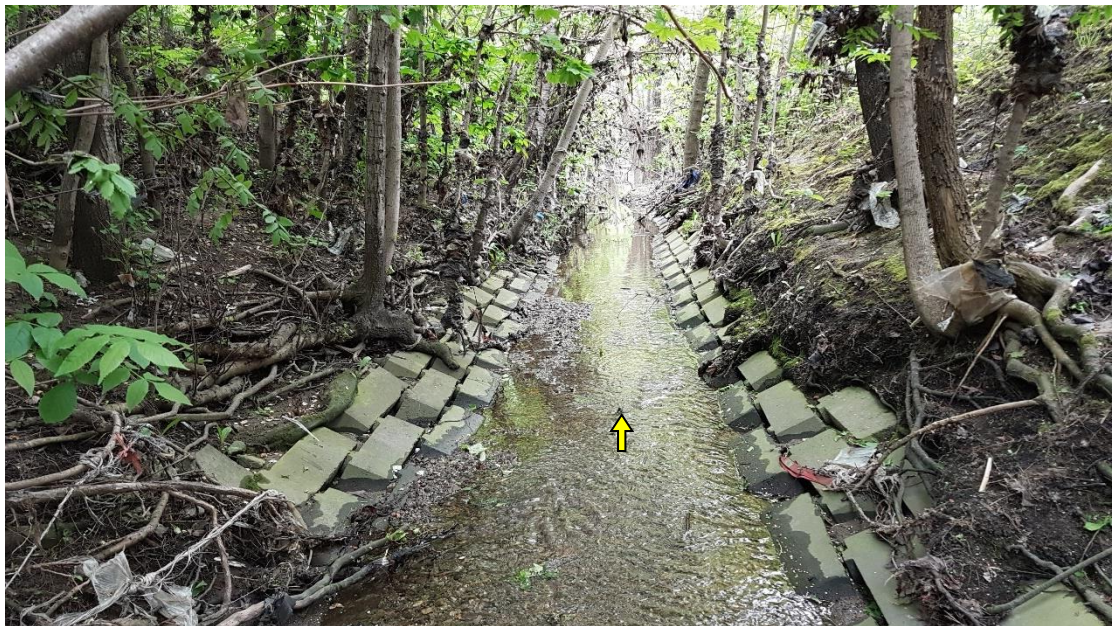
The entire length of channel and bank toe was underlain with an interlocking brick treatment, which had failed (e.g., dislodged) at multiple instances throughout the reach.
