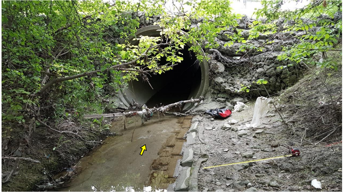
The Rutherford Road crossing consisted of a 1.9 m concrete culvert flanked by slumped gabion basket retaining walls.
